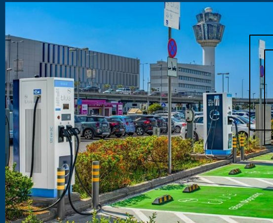
EV charging station
