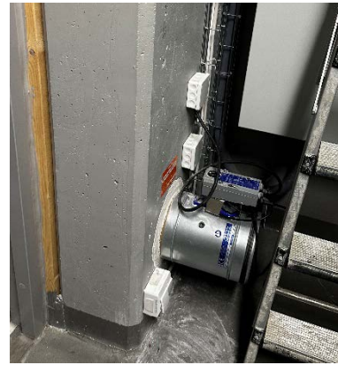
Fig. 8. Ventilation supply at floor level inside the battery room.
