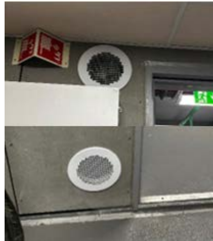
Fig. 9. Ventilation supply and extract at ceiling and floor level, seen from outside the battery room.
