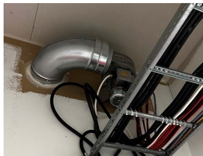
Fig. 10. Exhaust fan at ceiling level.
