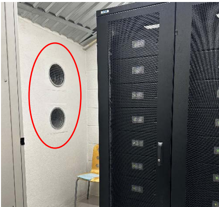
Fig. 2. Ventilation system, inside view. Air supply and extraction ducts shown with red circle.
