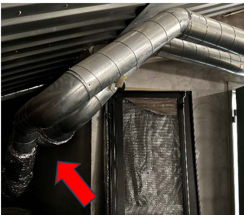
Fig. 3. Ventilation ducts, outside battery room, connected to main ventilation system. Air supply and extraction ducts from battery room marked with red arrow.
