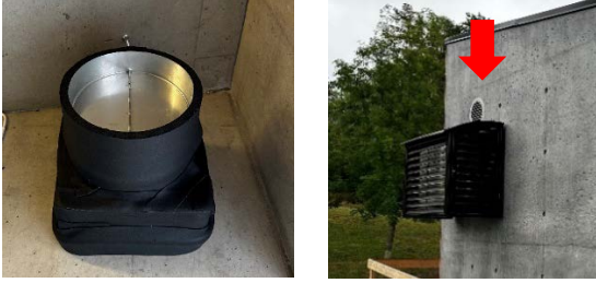
Fig.1. Right: Deflagration vent, inside battery room., Left: Deflagration vent, outside view, shown with red arrow.
