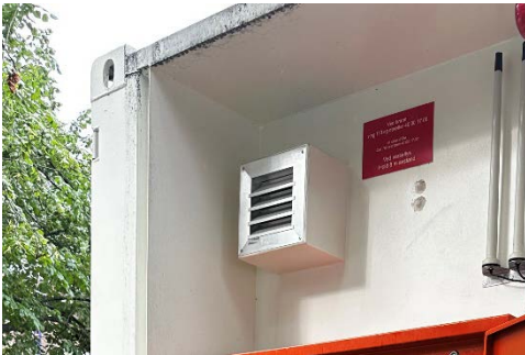
Fig. 6. Exhaust fan, seen from outside the container.
