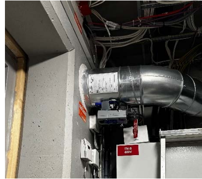
Fig. 7. Ventilation extract inside the battery room.
