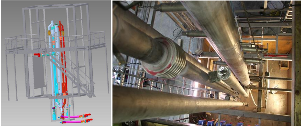
Left illustration: Planned layout of the CLC test rig Right photo: The CLC test rig from the top and down (Source: SINTEF)
