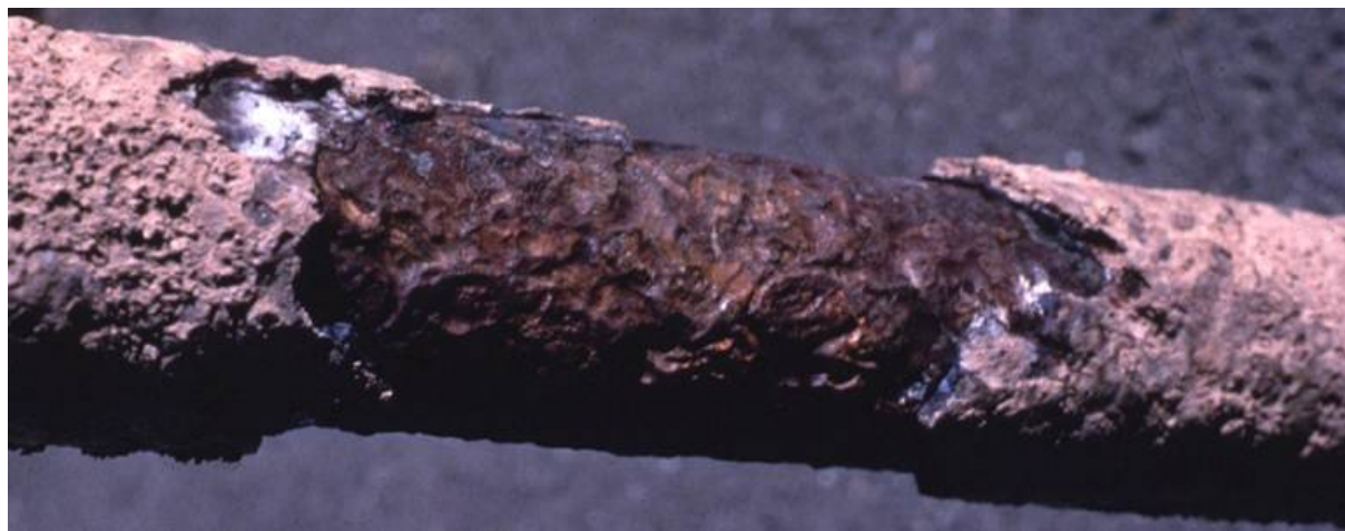
Figure 14: Corroded superheater tube from a biomass boiler (jenkins.ucdavis.edu).
