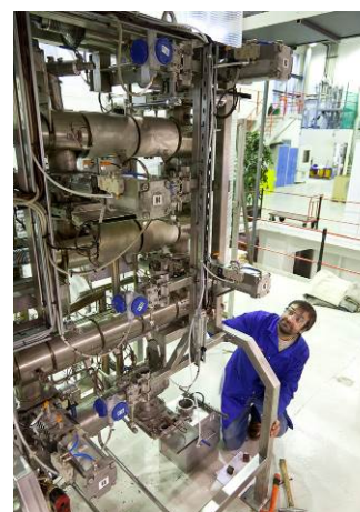
Torrefaction unit in Trondheim
