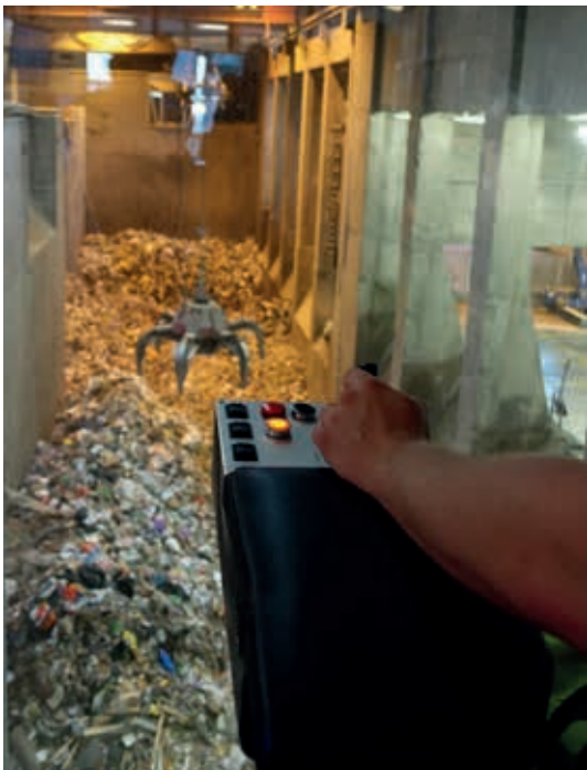
Waste-handling crane in operation in Statkraft Varme's Waste-to-Energy plant in Heimdal.
