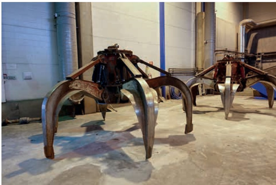
Waste-handling cranes at Statkraft Varme’s Waste-to-Energy plant in Heimdal. Photo: Alexis Sevault.
