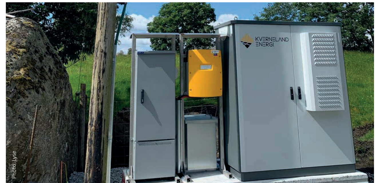
The system consists of an outdoor battery housing that provides voltage support to a small 230V overhead grid that supplies low voltage at certain periods.
