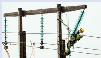
Sensor installation at Arva
