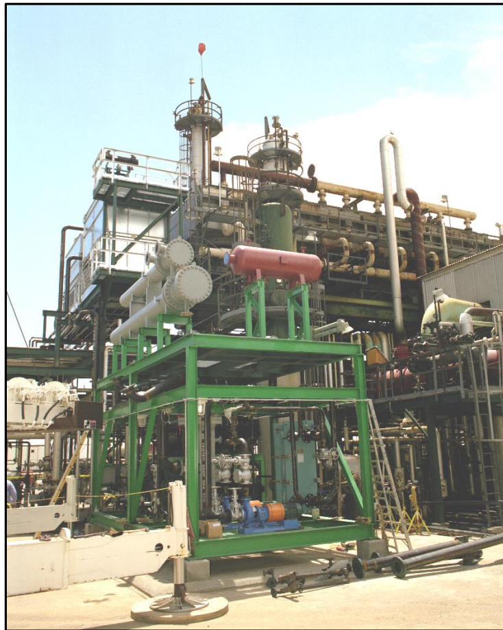
750,000 tonne/year ammonia plant using by-product hydrogen opens in Freeport, TX (2018; Yara, BSF)
