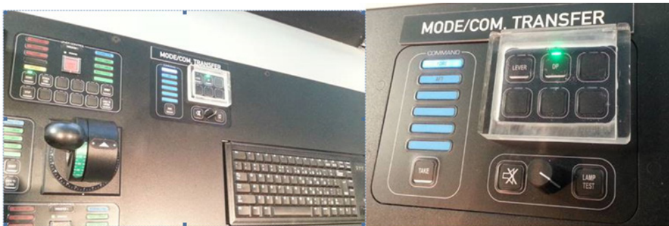
Figure 3: Close ups of (left) a manual lever control and the riser management desk, and (right) the utility panel with a protective Perspex cover fitted after the incident.
