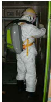
<Self-contained air unit>
