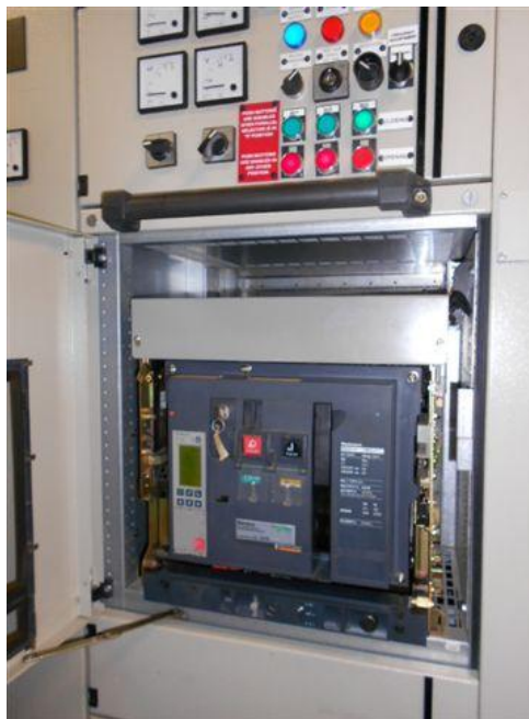
Switch nr. 901 (picture taken from Costa Favolosa)
