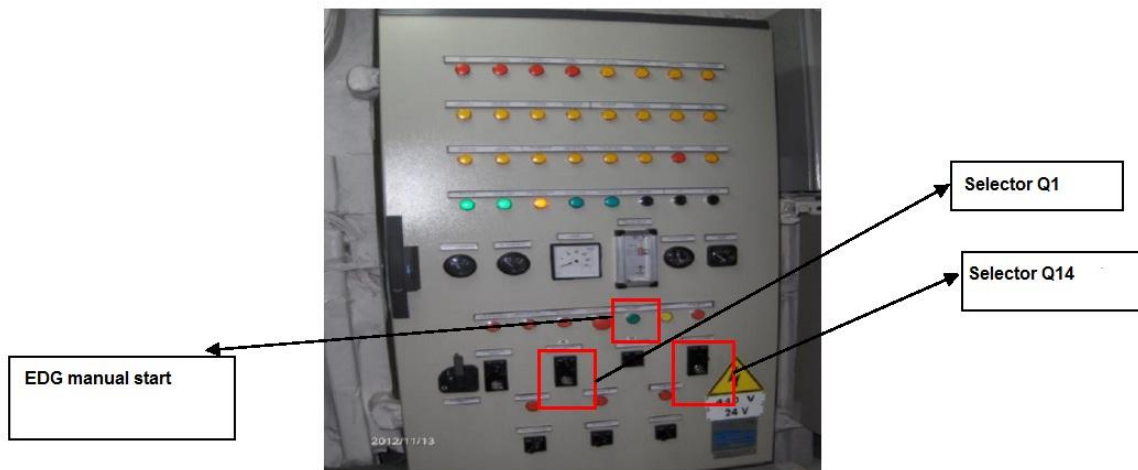
EDG switchboard (Part Number 1Q345063 – item mark XM/277 – sister ship Costa Favolosa)
