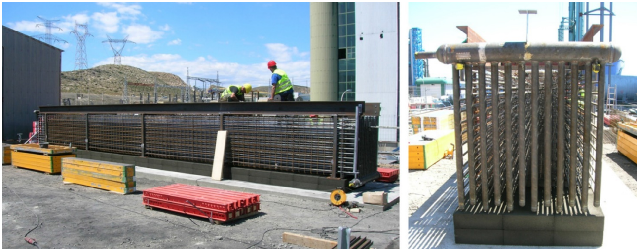
Figure 2-7: Tube register and collectors before pouring heat storage concrete (Laing, Bahl et al. 2011).
