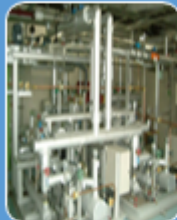
CO 2 cascade heat pump system with dry-ice sublimation
