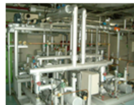
CO 2 Cascade refrigerating system
