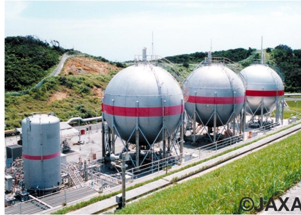
Rocket Base for JAXA (LH2 tanks, supply system)
