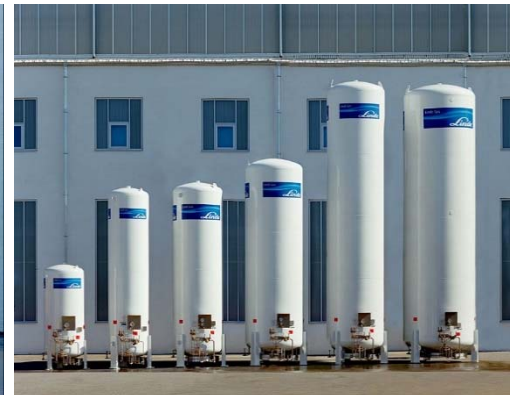
Cryogenic Storage Tanks
