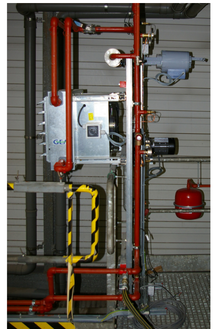
Ecoprobe cooling circuit installed at ISVAG (Belgium).
