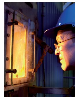
Visual control of combustion.
