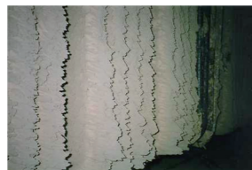
Deposits on a superheater formed by the combustion of waste wood. Photo: By courtesy of Vattenfall AB
