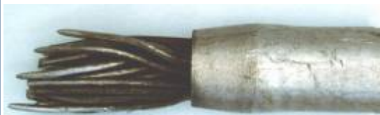
OH joint damage due to increased current
