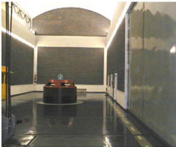
Figure 1. Inside Trollheim Power Station
