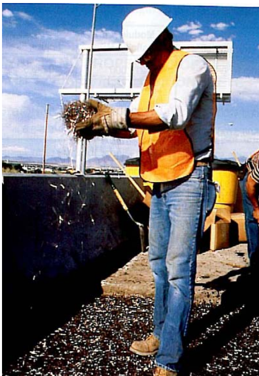
Figure 18: Placing of steel fibres before cement slurry is added in order to produce slurry infiltrated steel fibre concrete (ACI 544.1R-96 1997).
