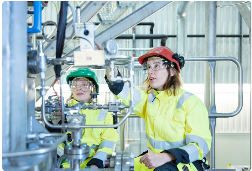
↑ Franziska Kausch and Judit Sandquist with the gasification reactor at SINTEF Energy Lab.
