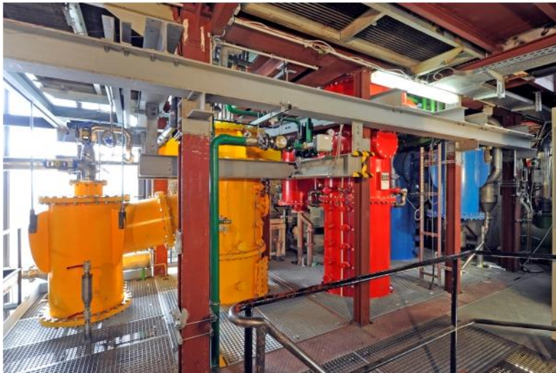
Alstom Power Calcium Looping – TRL 3
