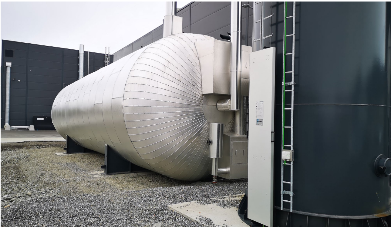
Steam accumulator at the Norsk Kylling plant in Orkanger.
