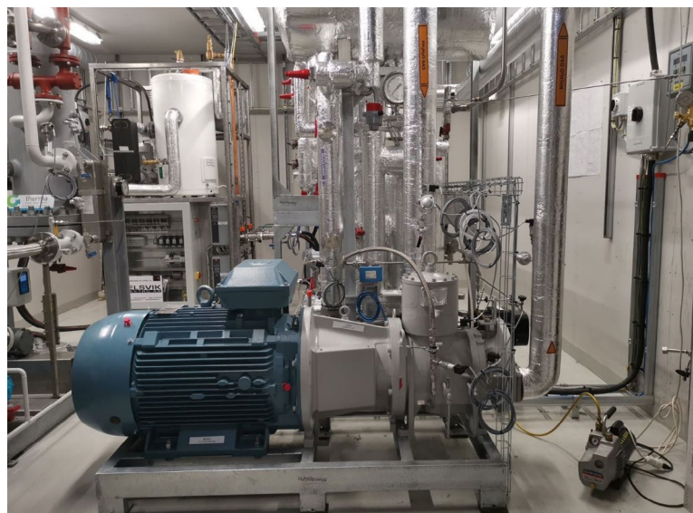
View of the installed combined absorption-compression heat pump test rig.
